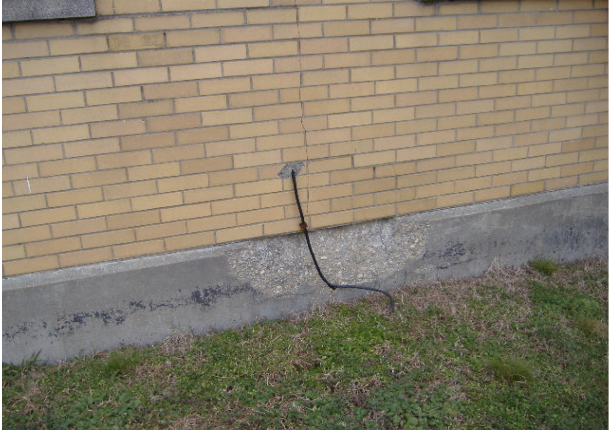
Floor slab spall.
