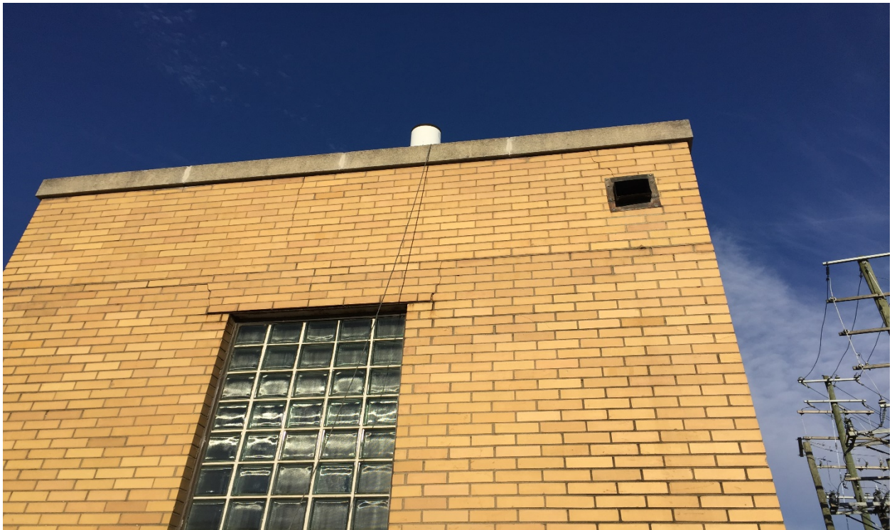
Cracking of brick at lintel bearing areas.
