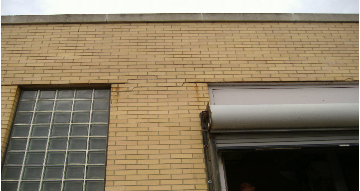
Cracking of brick at lintel bearing areas.
