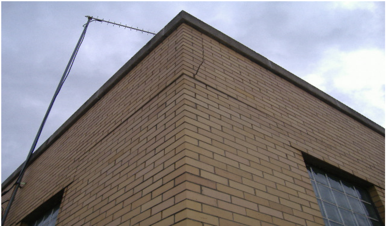
One of two corners where brick has pushed out along a bed joint. Also, cracking can be seen at the lintel bearing areas at the openings.
